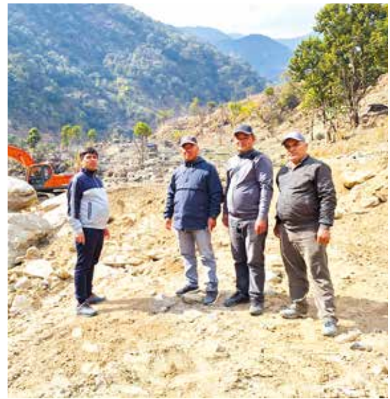
Damaged Khet Clearance at Rudi B HW area
