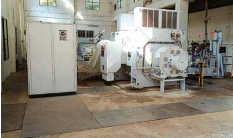
Power House Operating Area
