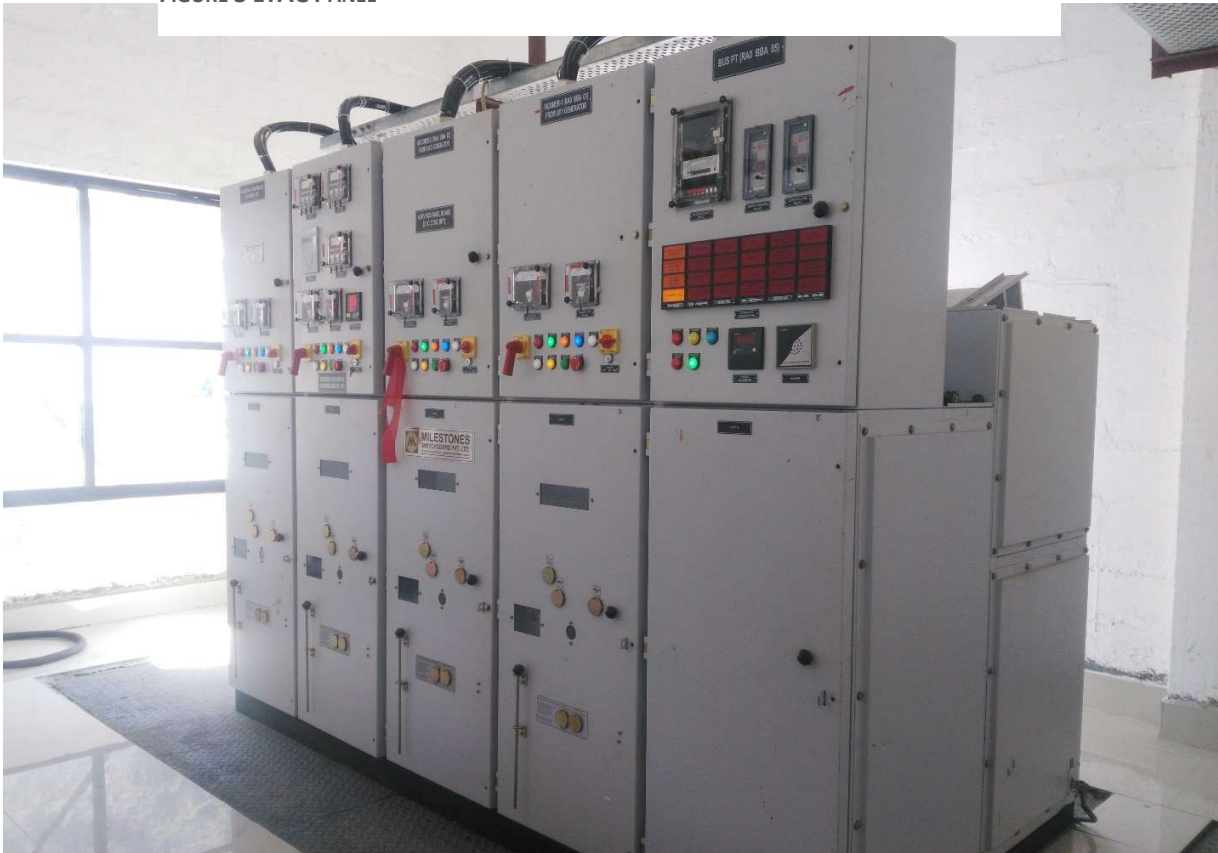
FIGURE 4 MV SWITCH GEAR PANEL
