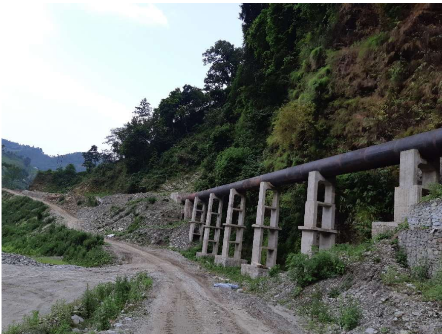
Fig 10: Headrace pipe section between AB-38 to AB-39
